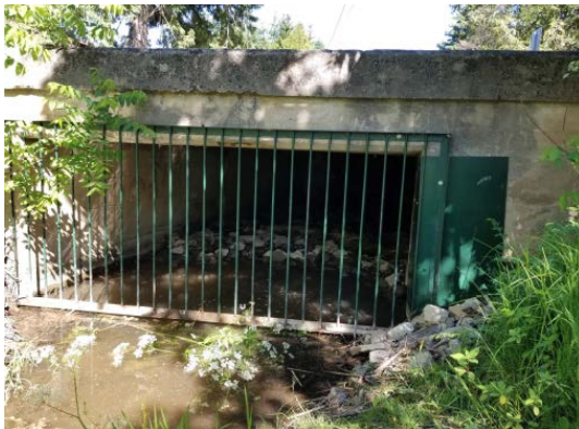
Figures 19 & 20: Culvert with BCI rating of 8
