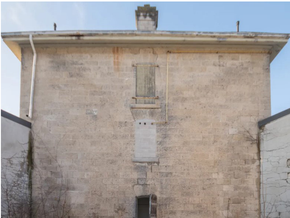
Figure 6.46 Exterior view of the existing conditions of the Jail Building facade from the exterior yard.
