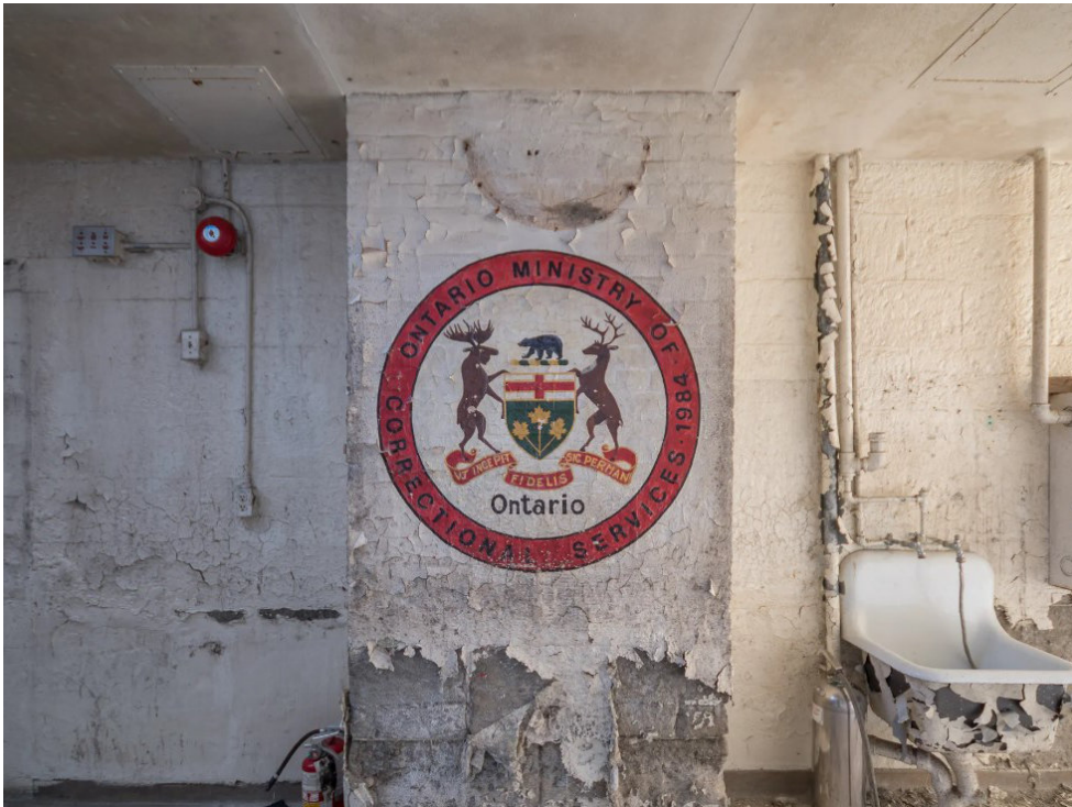
Figure 6.37 Interior view of the Jail Building Detail at the ground floor entrance.
