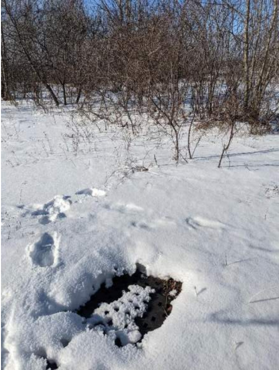
Photograph 10: Storm sewer grate found in the northwest corner of the property, looking northeast (January 21, 2022).
